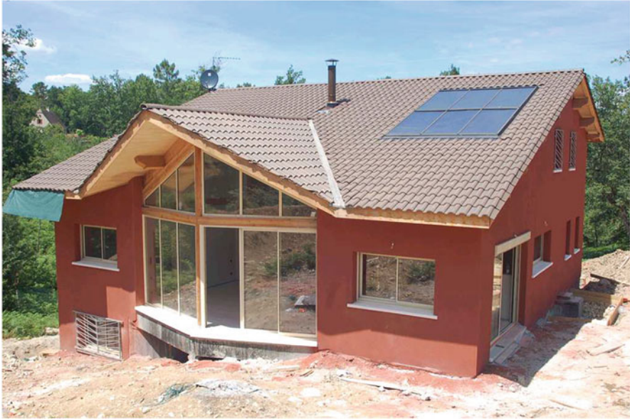
Fig. 6.1 View of the south façade of a 2-floor single-detached house located in south west of France. (From Moujalled et al. 2018). The walls are made of 30-cm thick coated sprayed hemp-lime concrete supported by a timber frame structure
