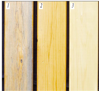
Fig. 2. Condition of samples with “Intol” fire retardant varnish after 10 years of exposure in the open air: 1 - on the test bench at an angle of 45°, 2 - on the wall, 3 - control.
