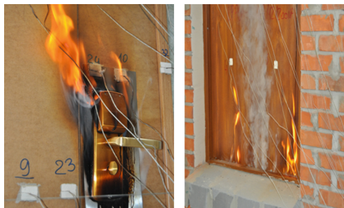
Fig. 1. Example of improper hardware (on the left) and lack of suitable intumescent seals (on the right).
