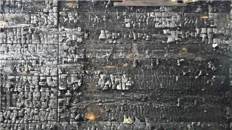
Fig. 2. CLT panel that has been fire tested and is showing char fall off (image, Arup)
