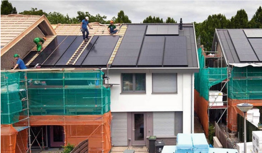
Fig. 9.7 Installation phase of the prefabricated elements of the building envelope in a residential building in UK, within the Energiesprong project. Credits The Renewable Energy Hub, https://www.renewableenergyhub.co.uk/blog/what-are-energiesprong-homes/
