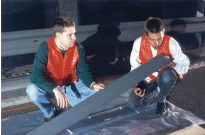
Fig. 3 CFRP laminates are going to be prepared for the application on the soffit of the Ibach Bridge
