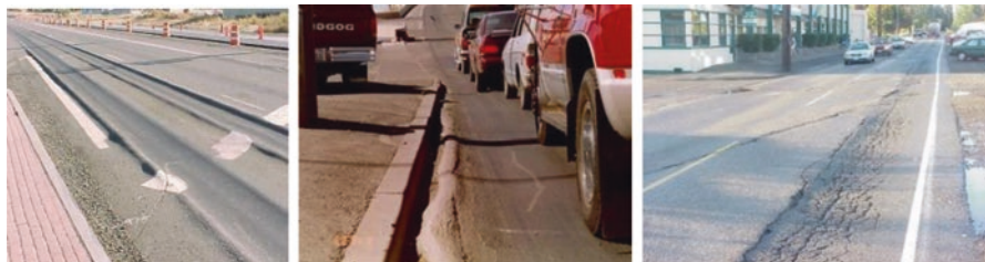
Fig. 1 Severe mix rutting (left), mix rutting (middle), and rutting in the wheel path (right) [3]
