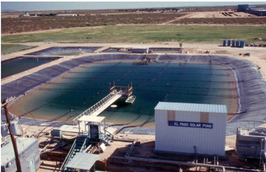
Fig. 3.28 A model of a desalination plant operating in a multi-stage flash evaporator through a solar pool (El Paso station) (University of Texas at El Paso 2002)
