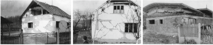
Fig. 3.6 Damages of residential houses caused by Banja Luka 1969 earthquake (Stojković 2009)
