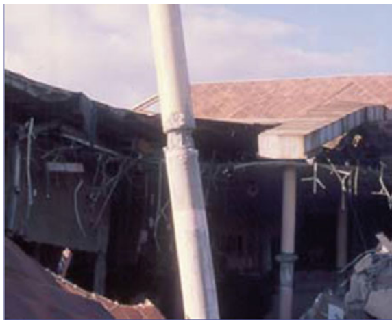
Fig. 6.8 Damage to the slab due to the punching of the column through the foundation (Wallace et al., ND)
