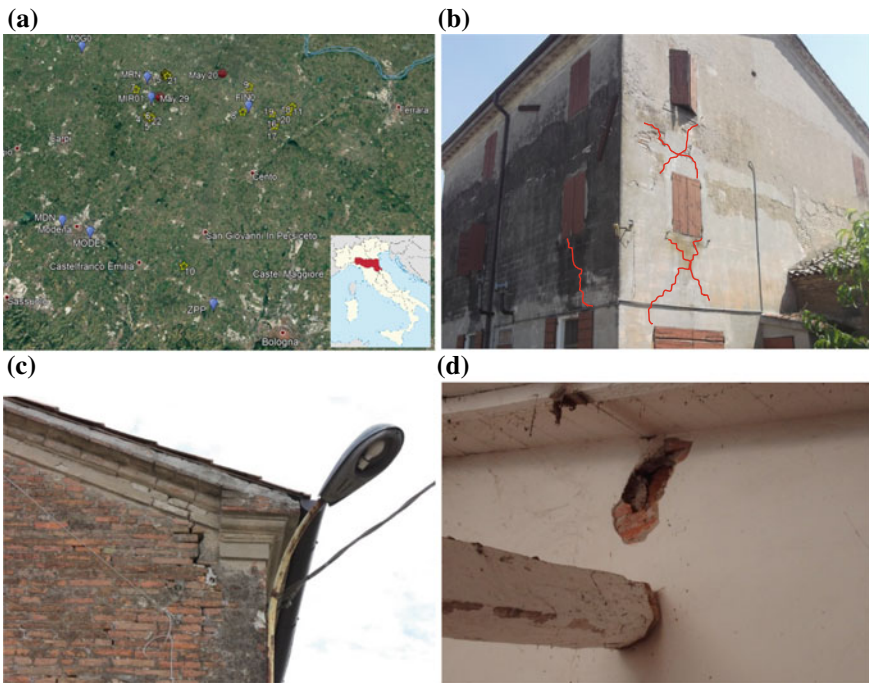
Fig. 1 View of the area stricken by the Emilia earthquakes with a localization of buildings and damage to residential buildings: b cracks on masonry wall; c corner damage; d fall of a wooden beam
