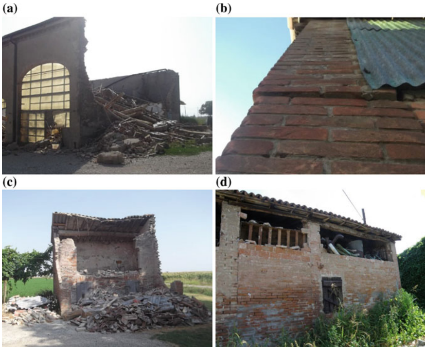
Fig. 3 Main damages to buildings used for minor services
