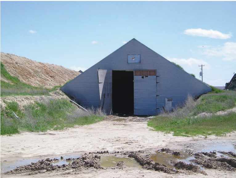
Fig. 17.1 For decades, commercial potato production has used many kinds of storage structures. Older storages lacked all but the most basic climate controls
