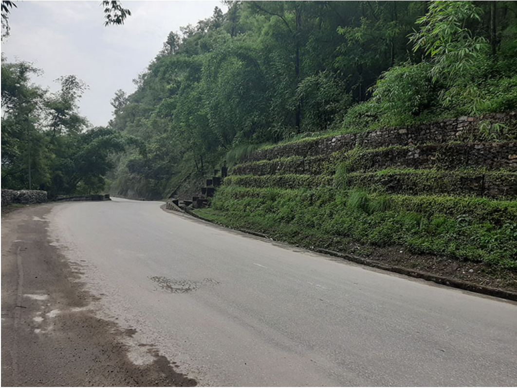
Fig. 9.5 Low-cost mitigation measure in Krishnabhir Landslide at Prithi Highway connecting Kathmandu and Pokhara. The gabion retaining wall and associated bioengineering have helped to reduce the likelihood of slope disasters on this particular section of the landslide. Credit Ranjan Dahal
