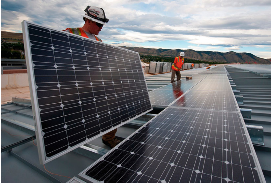
Fig. 8.1 Installation of solar panels as part of sustainable building practices. Image by skeeze from Pixabay
