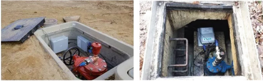
Fig. 12.9 Monitoring water mains through smart acoustic correlators linked to GIS. Courtesy Echologics and Mueller Co. [19]
