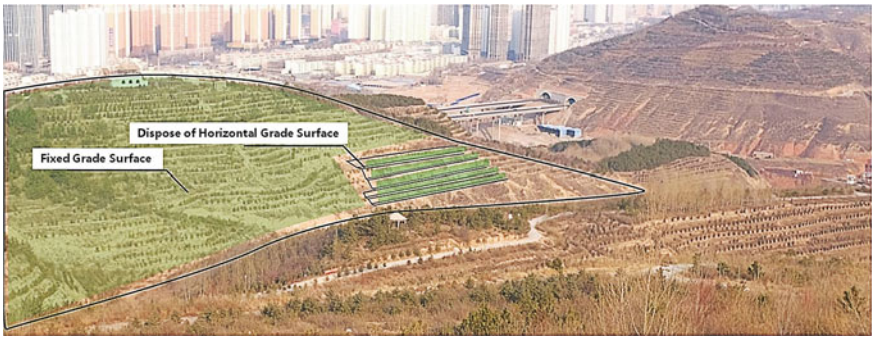
Fig. 5.19 Illustration of the construction of the exposed mountain sponge facility. The image demonstrates the layout of some stormwater facilities such as terrain remediation and setting up gullies to collect rainfall flows on site (Source Xining Forestry Bureau 2015)
