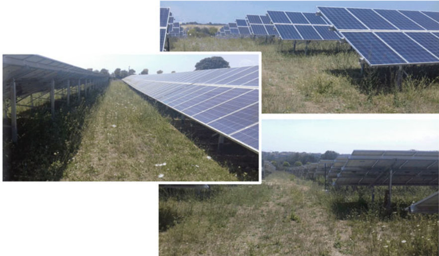
Fig. 1 Pictures of the 2 MW PV plant in Central Italy that represents the case study of this work
