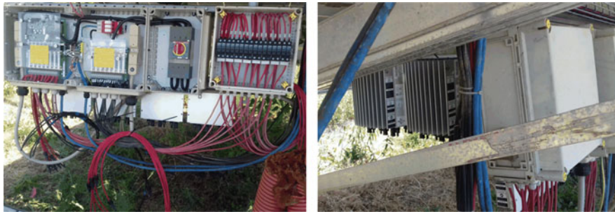
Fig. 2 Photos show the mounting of the string optimizers. Left: cabling modification at the string box. Right: string optimizers mounted at the rear side of the string box
