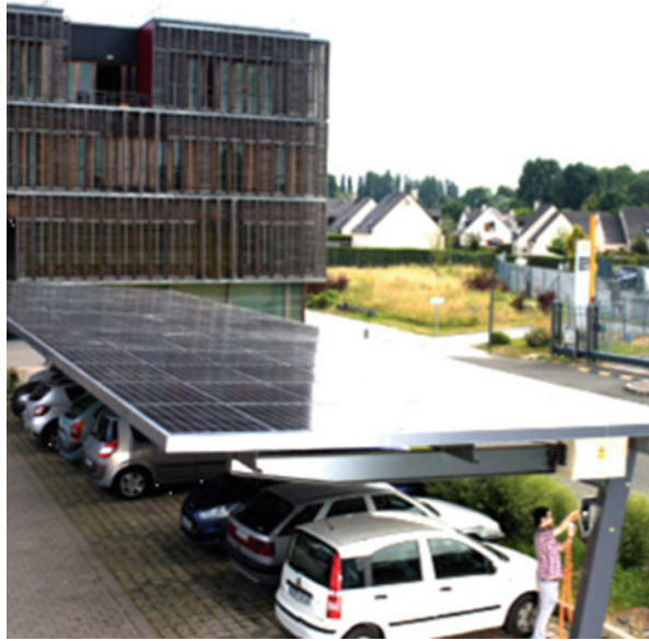
Fig. 1 Photovoltaic panels in the campus in Compiègne, France
