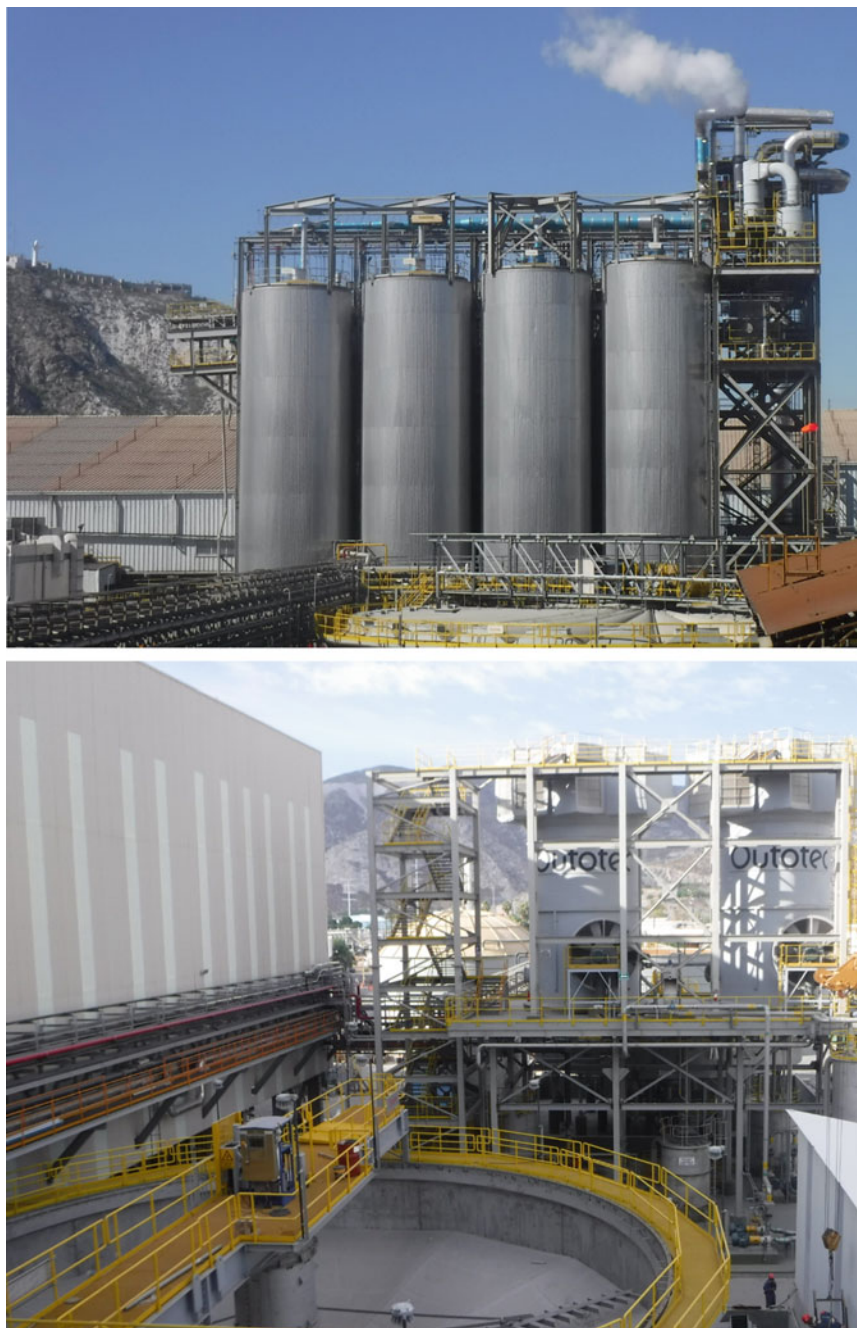
Fig. 2 DL reactors with off-gas treatment (upper) and Cl removal thickener and gypsum removal cooling tower installations close to the new solution purification building (lower)
