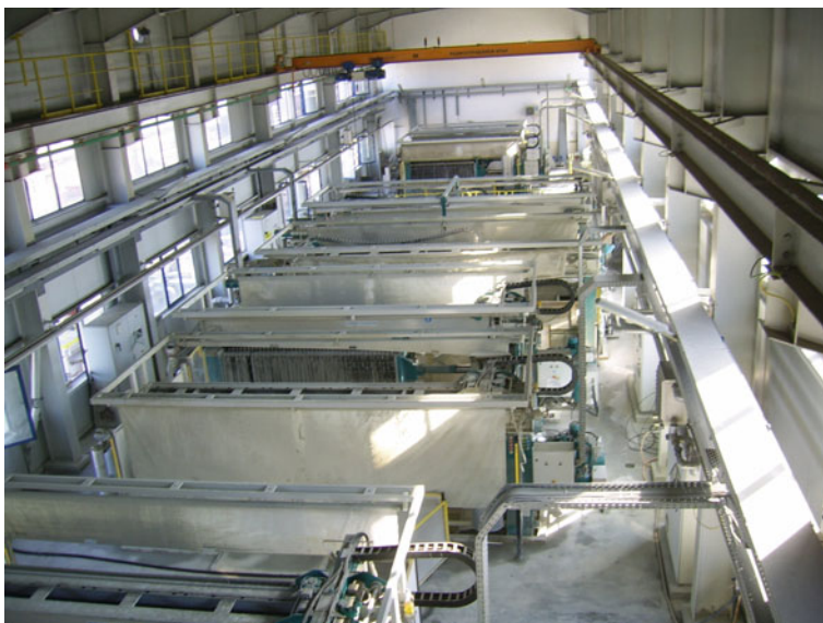
Fig. 3 Installation for washing and leaching of Waelz oxides—filtering department
