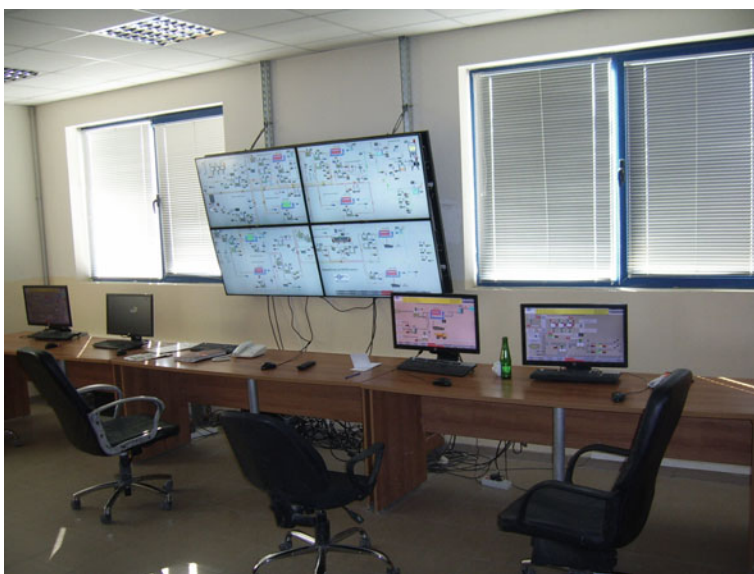
Fig. 4 Installation for washing and leaching of Waelz oxides—control room
