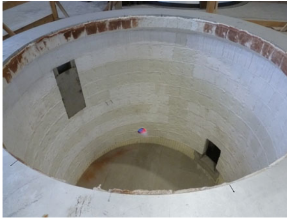
Fig. 7 Lining of a kettle station with openings for maintenance and the burner equipment
