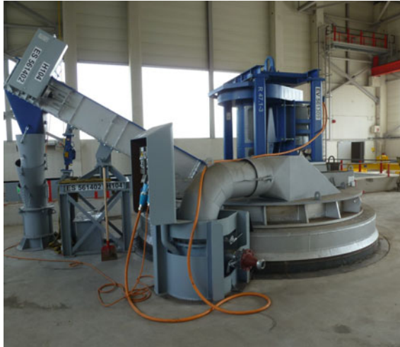
Fig. 4 Sealed kettle with an installed stirring device, an access point for a dross removal equipment (drag chain conveyor) and the connected duct to the secondary ventilation
