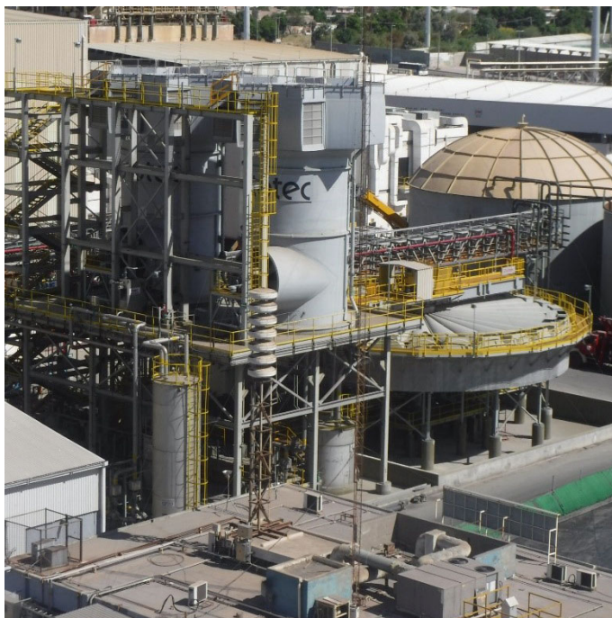
Fig. 1 Gypsum removal circuit in Torreon. 2pcs of Outotec cooling tower 6000 and an Outotec high rate thickener
