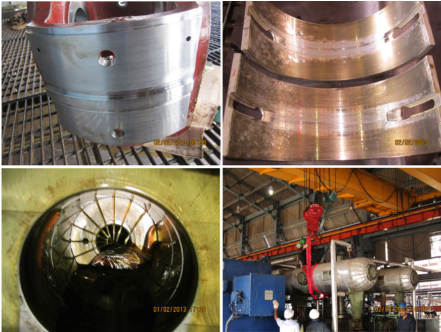
Fig. 12 Parts of MUG Compressor showing marks of damage
