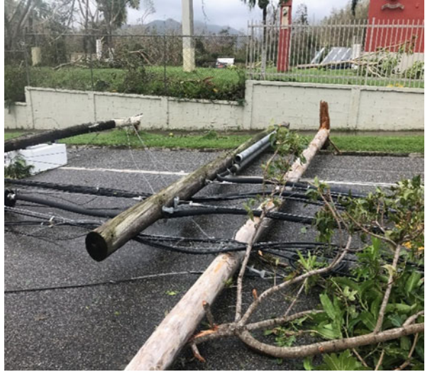
Fig. 2 Terrestrial infrastructure can struggle to withstand the forces of nature. (Graphic courtesy of Hughes Network Systems)
