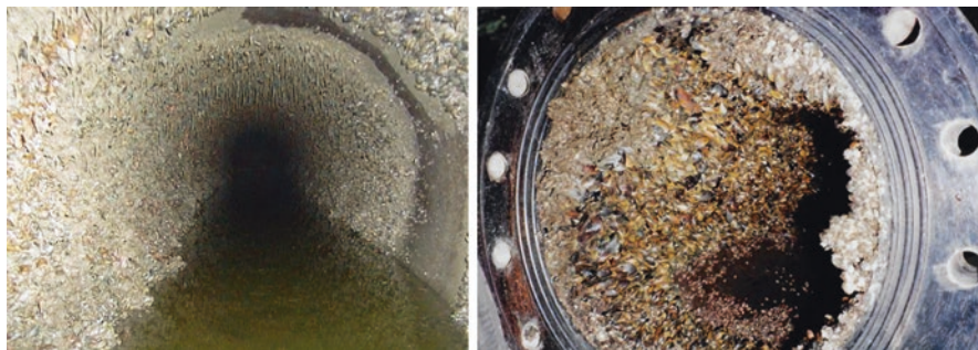
Fig. 16.4 Biofouling in sea water intake pipelines and headers. (Source: H2O Biofouling Solutions B.V.)
