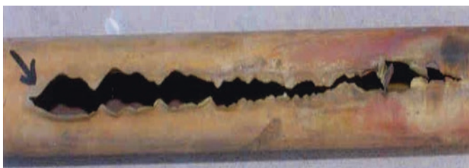
Fig. 5.10 Erosion-corrosion of Al brass tube from a MED plant
