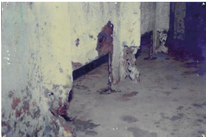
Fig. 5.5 Severe erosion-corrosion of carbon steel in MSF flash chamber structure
