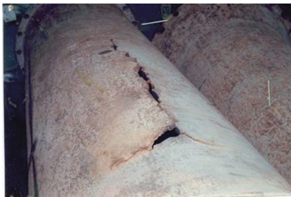
Fig. 5.6 SCC of Ni-resist D2 in brine recycle pump column
