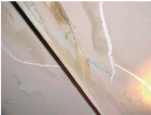
Fig. 5.19 Cracks on the welds of the bottom stiffeners from distillate tray
