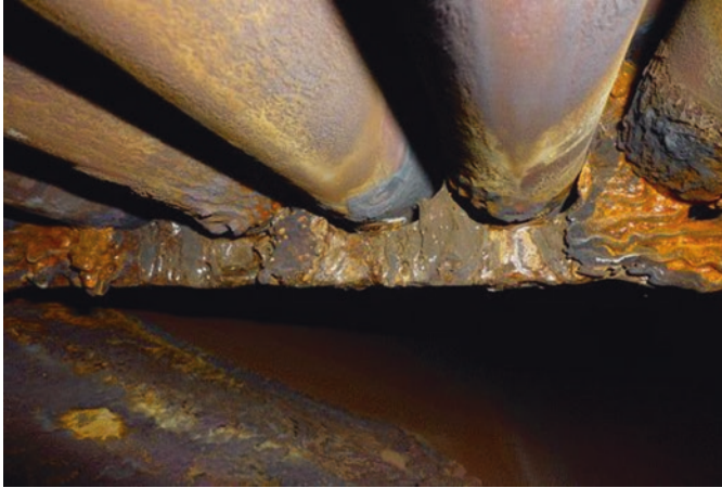
Fig. 5.13 Galvanic corrosion between tube and tube baffle in MSF plant
