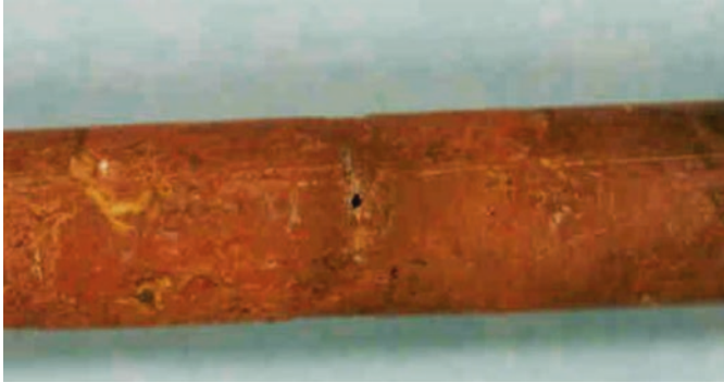
Fig. 5.11 Pitting corrosion on MSF condenser tube from 5th stage after 13 years of operation
