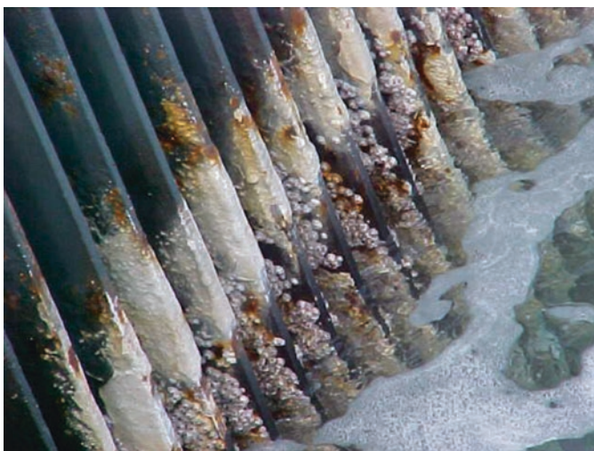
Fig. 5.18 Splash and crevice corrosion caused by barnacles attachment on bar screen in desalination intake
