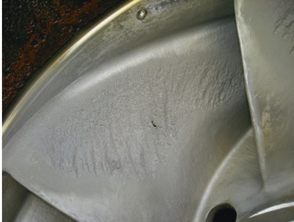
Fig. 5.20 Cavitation on brine recycle pump impeller after 19 years of service
