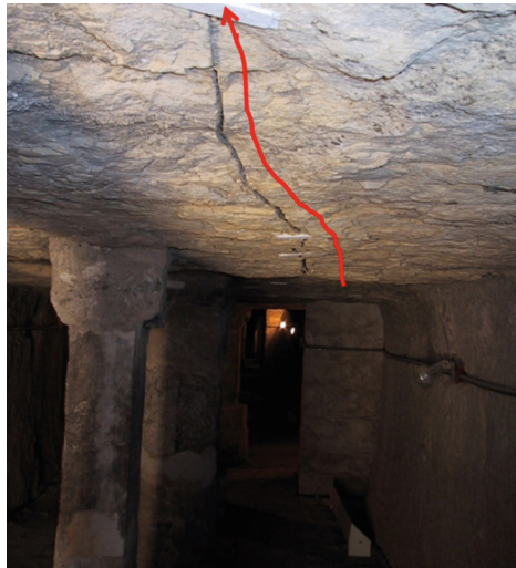
Fig. 4. The critical state of roof layers in the southern entrance roof– level 1
