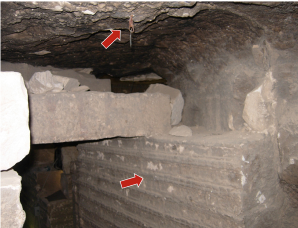
Fig. 11. Gallery ceramic panel, partial failure
