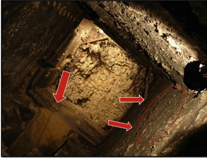
Fig. 5. Burial shaft failure zone
