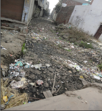
Fig. 2. Shows drains at Jamalpur, Aligarh.
