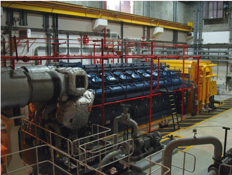
Fig. 18.2 Essential diesel and generator
