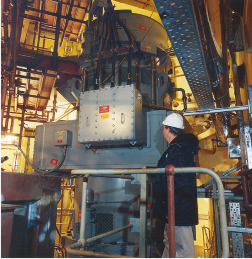
Fig. 6.8 A reactor coolant pump (RCP) motor
