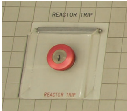
Fig. 11.1 The Reactor Trip Button
