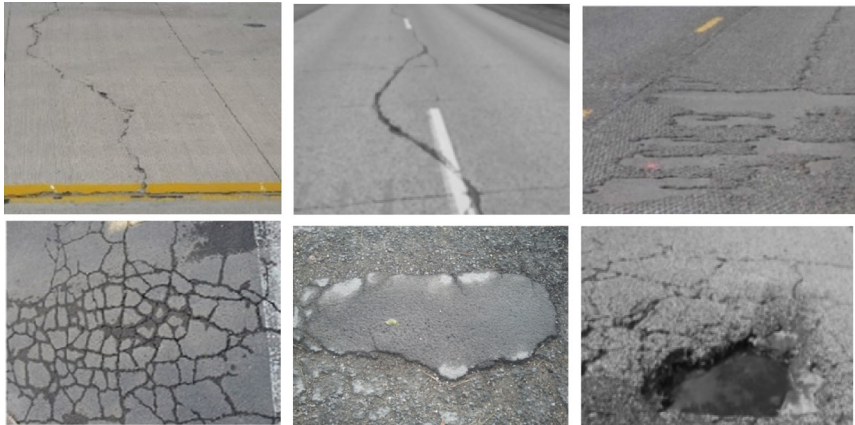
Fig. 1. Examples of structural damages typically found in the literature: (a–b) linear cracks, (c) peeling, (d) alligator cracks, (e) patches and (f) potholes
