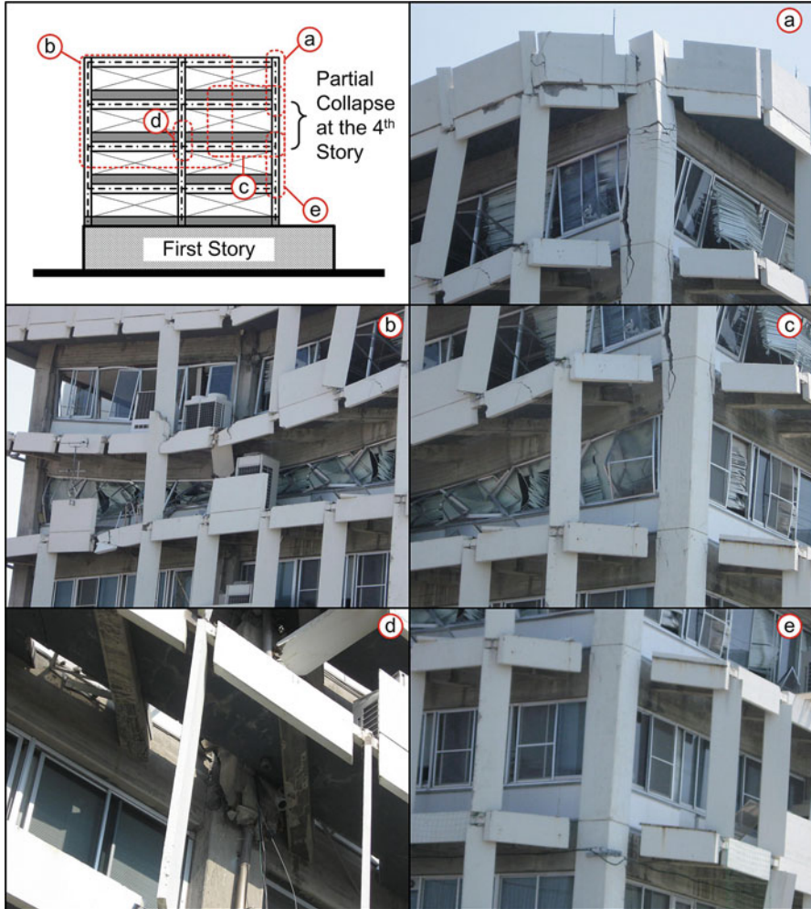
Fig. 32.5 Simplified elevation and photographs of the west elevation. Photographs show (a) damage to the corner column on the fifth story, (b) partial collapse of the fourth story, (c) damage to the corner column on the fourth story, (d) damage to the bottom of a fourth story, and (e) damage to the corner column on the third story
