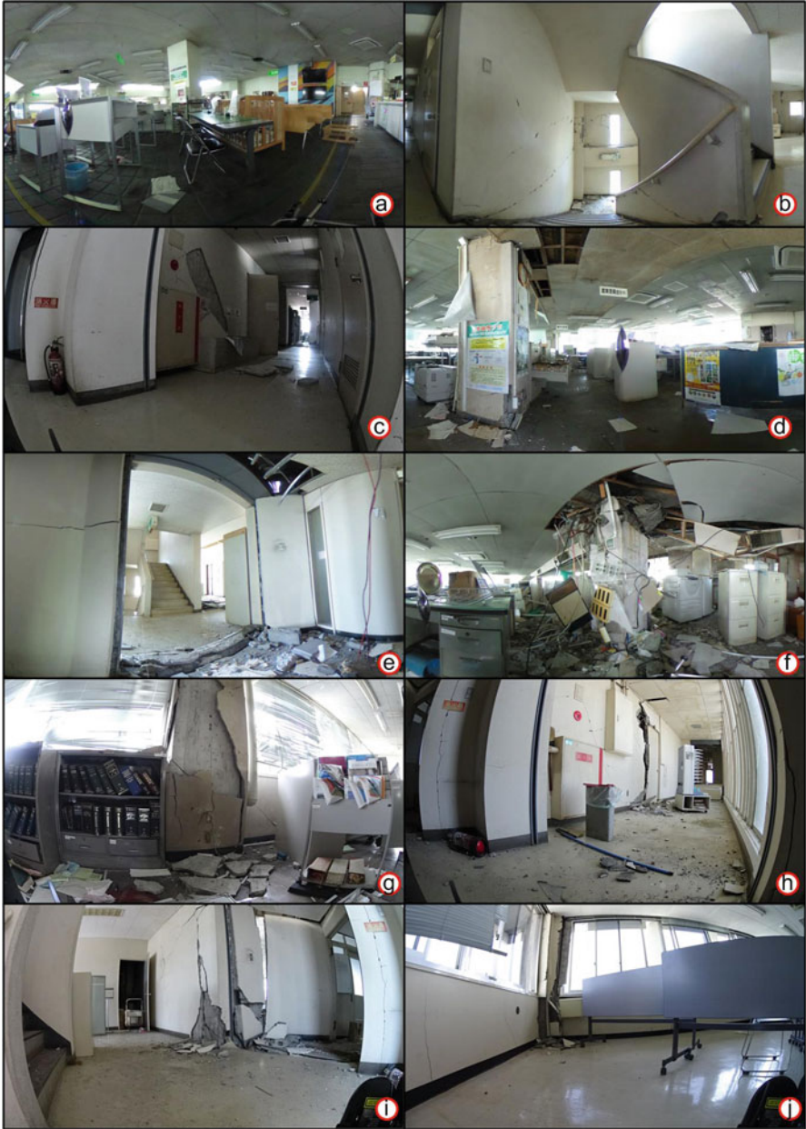
Fig. 32.9 Photographs of the damage taken by the robot inside the main building of Uto City Hall. The locations from which the photographs were taken are shown in Fig. 32.8
