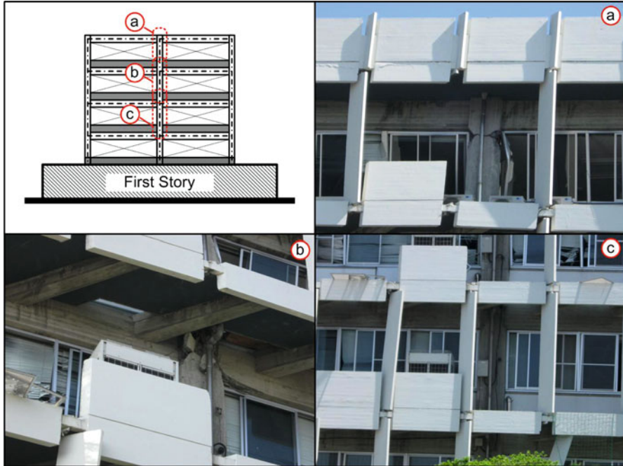
Fig. 32.4 Simplified elevation and photographs of the south elevation. Photographs show damage to (a) a fifth-story column, (b) a beam–column joint at the top of the fourth story, and (c) a third story column
