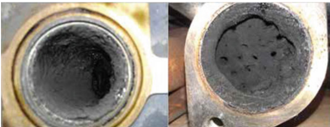
Fig. 5 Wet stacking—“extreme clogging” of exhaust pipe [5]
