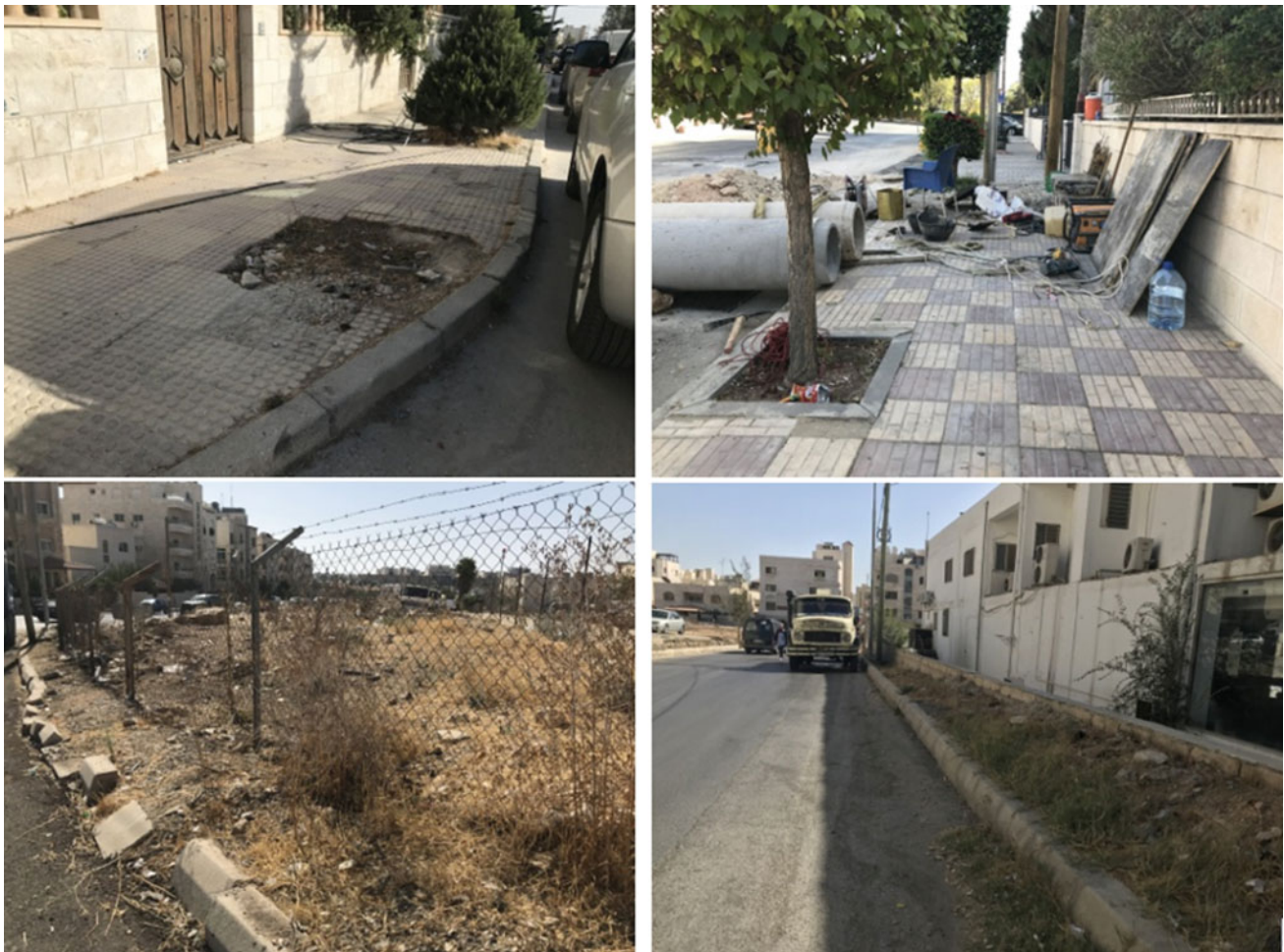
Fig. 5 Deteriorated sidewalk examples Source Author (2017)
