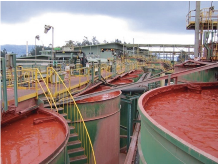
Fig. 5.2 Carbon-in-leach plant (Gorain et al. 2015)
