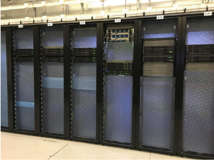
Fig. 4 EPIC's servers, switches, and routers for the network emulation
