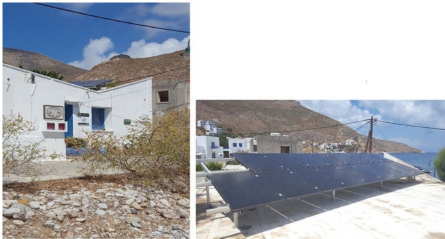
Fig. 31.7 PV Station at Tilos island
