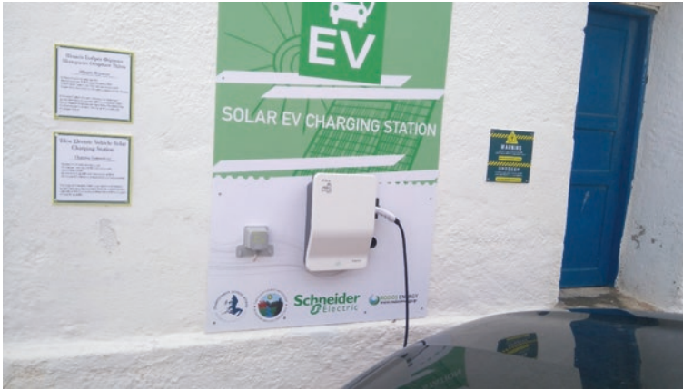
Fig. 31.8 Solar-based EV charging station in Tilos island
