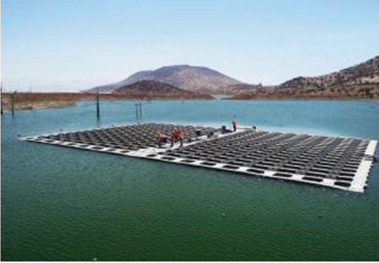
Fig. 27.16 Chile floating 84 kW, PV farm on lake north of Santiago supplying 153 MWh a year to the mining community at the beginning of 2019
