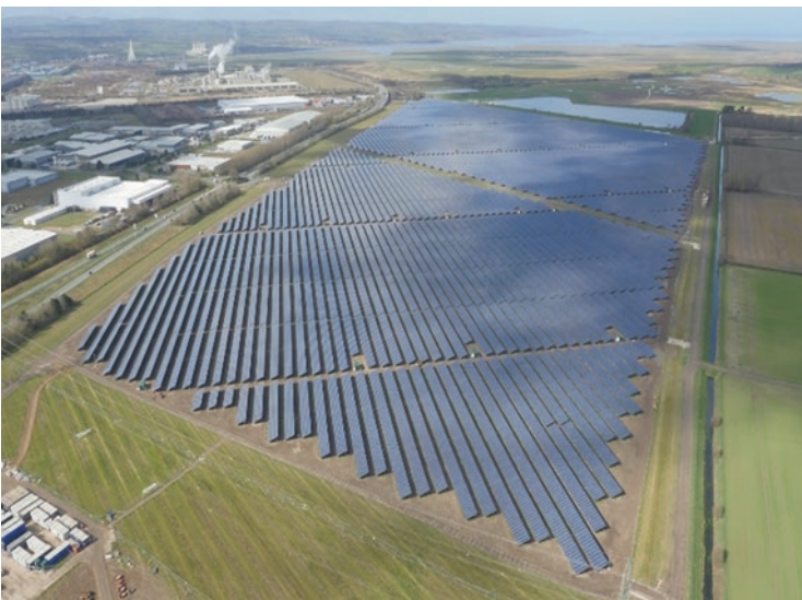
Fig. 43.6 The 50 MW Shotwick Solar Park
