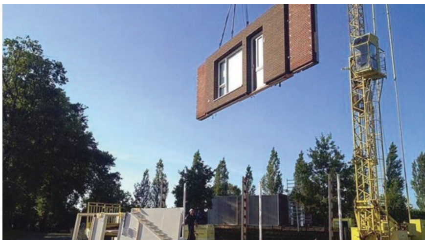
Fig. 22.2 Handling of the prefabricated panels according to the project of Ron van Erck for the energy requalification with prefabricated panels. Source: Centomila case riqualificate in 10 giorni, a Rebuild il super-sistema dell'olandese van Erck—by Mila Fiordalisi, Edilizia e Territorio—Sole 24 ore, 25 June 2015
