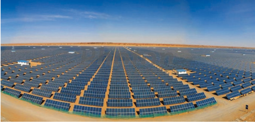
Fig. 27.13 Large PV installation in China
