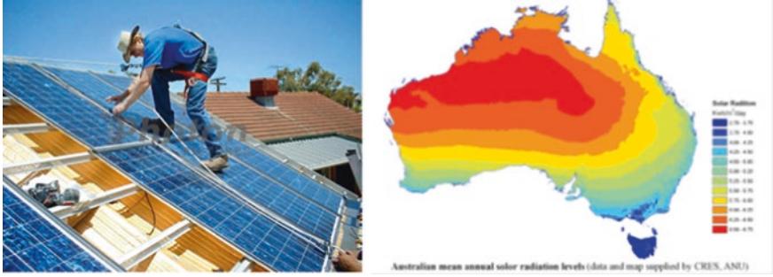
Fig. 27.9 Rooftop installation in Australia and Solar Radiation Map (4.00–6.75 kWh/m 2 /day) [11]
