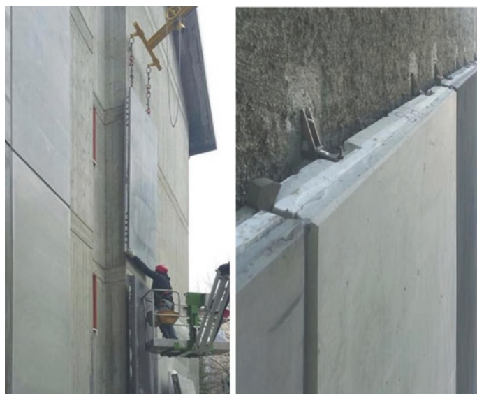
Fig. 22.6 Application of the insulating covering panels and detail of the wall anchoring system. Source: “Soluzioni prefabbricate per la riqualificazione energetica dell’involucro” by Graziano Salvalai, aZero n. 20, pp. 56–69—EdicomEdizioni
