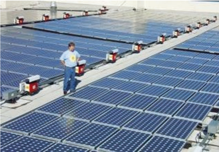
Fig. 27.14 Los Angeles Department of Water and Power (LADWP) plant
