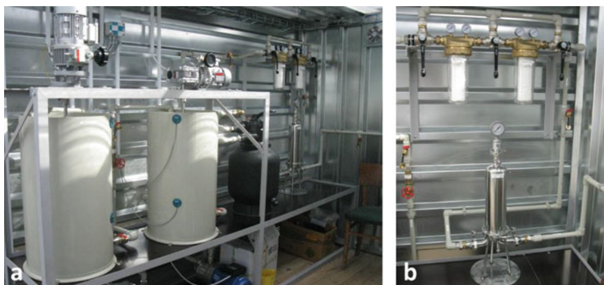
Fig. 13.4 (a) The overall view of the semi-pilot plant—mixing reactor, tank for ageing, sand filtration (the black container), two-phase microfiltration (in the top right-hand corner), ultrafiltration (the silver container below the microfiltration). (b) Detailed picture of microfiltration (at the top) and ultrafiltration (silver container below)
