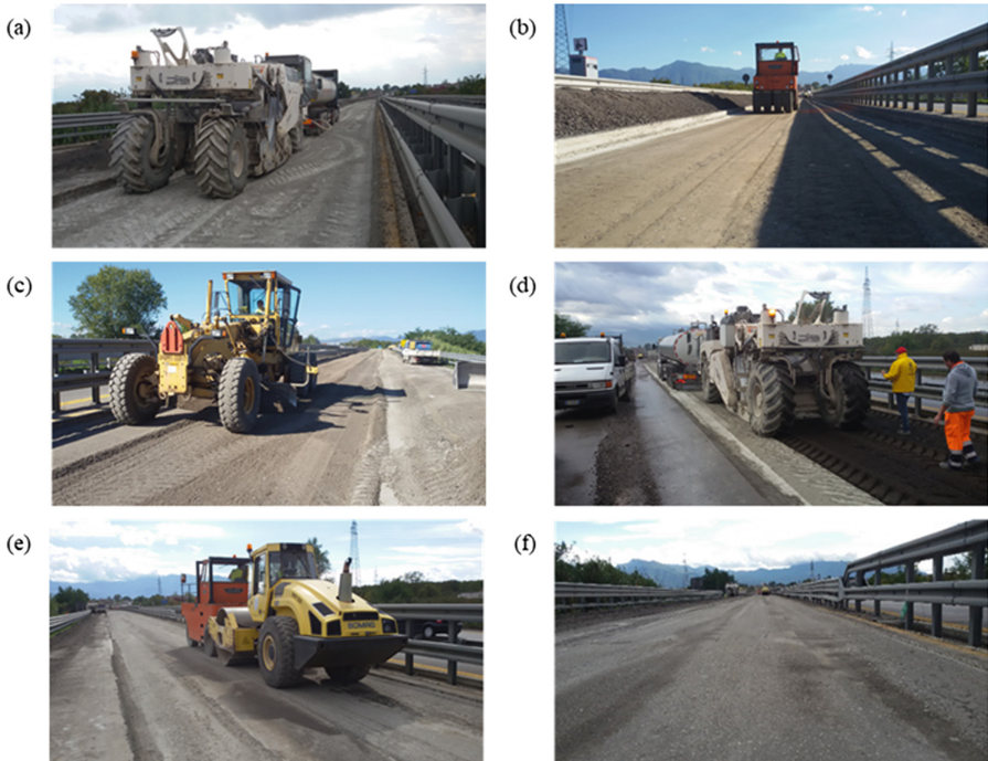
Fig. 1. Photos taken during the construction of the experimental pavement section: (a) first recycler pass for mixing CSF layer; (b) compaction of CSF layer; (c) levelling of the RA; (d) second recycler pass for mixing CRAB layer; (e) compaction of CRAB layer; (f) compacted CRAB layer before sealing.
