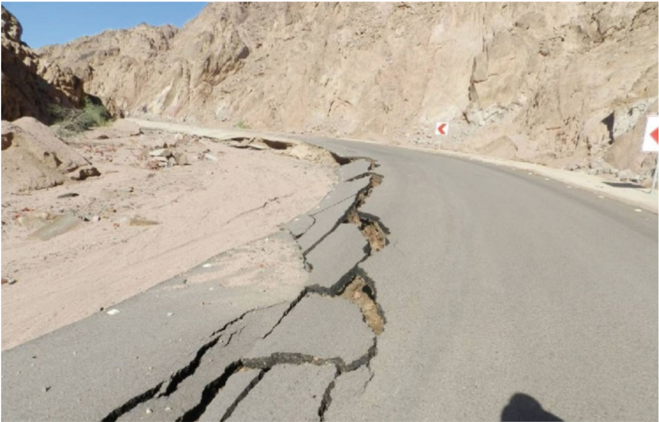
Fig. 5 A photo showing the destroyed main road to W. Dahab Watershed
