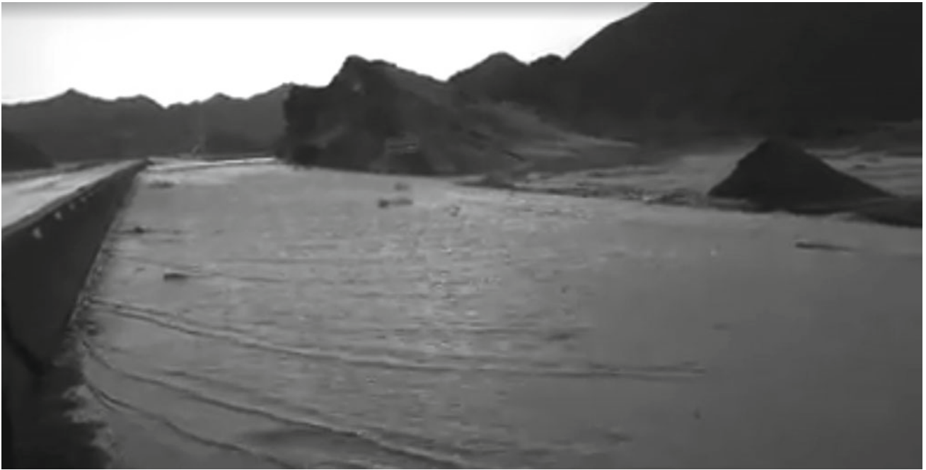
Fig. 10 Safaga-Qina road after April 12, 2017 rains
