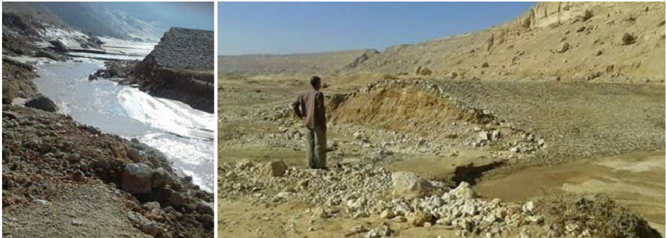
Fig. 16 Partial failure of Galawya dam due to the use of the dam top as an access road for quarries trucks (MWRI 2016)
