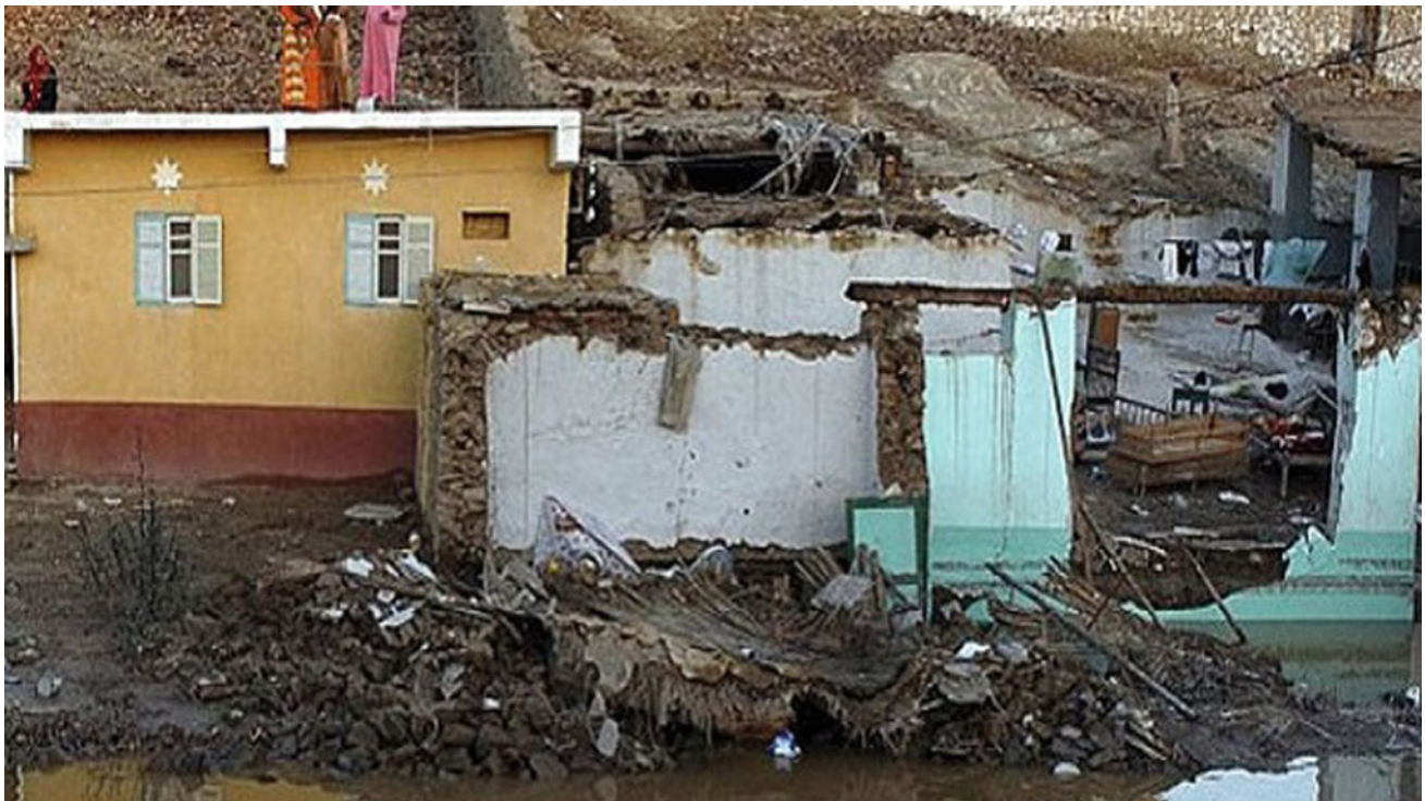
Fig. 7 Buildings are destroyed in Abouelreesh village in Aswan governorate after a torrent on June 17, 2010
