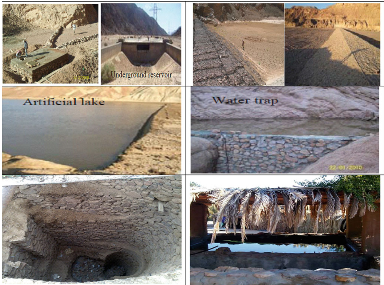
Fig. 6 Underground (Haraba) reservoir construction for water harvesting in Wadi Watier near Nuweiba City. a Low-cost gabions and obstacle dam constructed in Wadi Ghazala, b (WRRI 2010) artificial lake, c water trap, d well, e water storage tank, and f for water saving in Feiran Oasis
