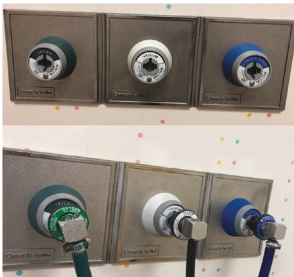
Fig. 4.19 Figure showing gas outlet panel of oxygen, nitrous oxide, and vacuum using DISS system
