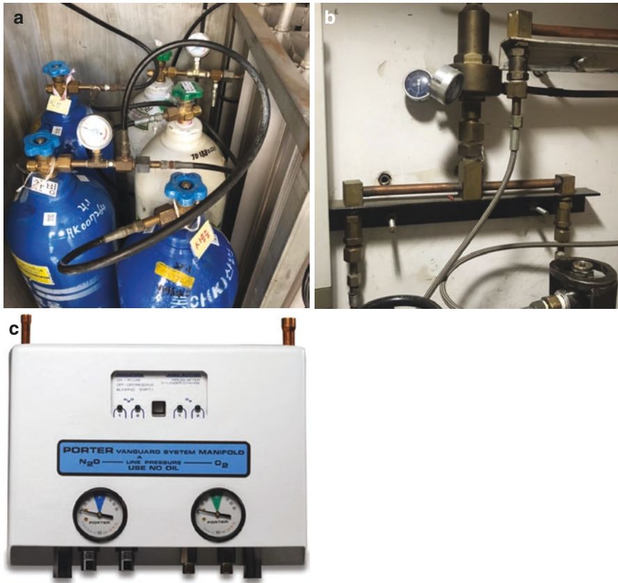
Fig. 4.17 (a) Conventional type of manifold attaching two cylinders of each gas with a separate cylinder pressure gauge for each gas. (b) Figure showing nitrous oxide manifold with pressure gauge and regulator. (c) Manifold by Porter Inc. showing in-built line pressure gauges and indicators for two cylinders each of nitrous oxide and oxygen. (Source: Porter Vanguard Manifold . https://www.porterinstrument.com/product/dental/Porter-Vanguard-Manifold )
