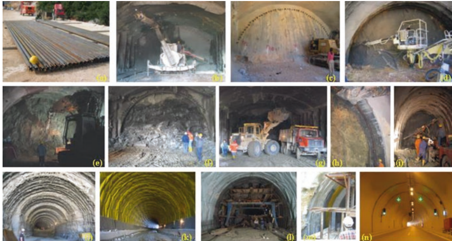
Fig. 21.10 Sequencing of tunnel construction at selected stages; (a) forepoles, (b) Installation of forepoles at tunnel face using forepoling machine, (c) view of tunnel face with forepole umbrella inserted, fiberglass dowels, and drainage pipes, (d) shotcrete being applied, (e) controlled excavation of face, (f) excavated material, (g) removal of excavated material, (h) installation of structural support—steel sets, (i) installation of further radial support—grouted rock bolts, (j) successive forepole umbrellas seen as well as bench, (k) installation of geomembrane, (l) installation of steel reinforcement for final lining, (m) detail of reinforced final lining, and (n) completed tunnel
