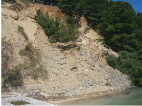
Fig. 12.2 Landslide at the sea coast on the natural cliff in flysch formation. Location: Split, Croatia
