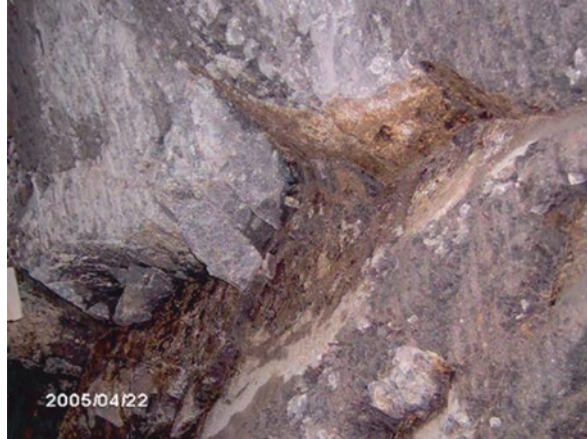
Fig. 20.5 Rock fall at Covão tunnel (Sousa 2010)
