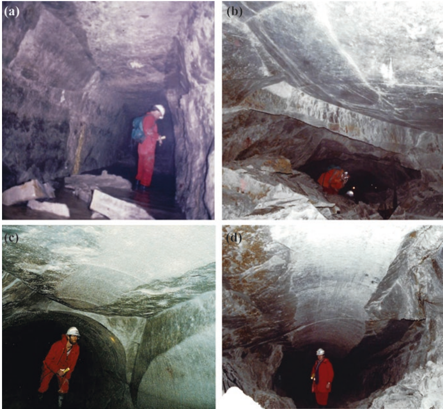
Fig. 18.4 (a, b) Joint and bedding plane controlled overbreak in Terlingham Tunnel and in Beaumont Tunnel. Some of the 2.2 m diameter tunnel can be seen in the background in (b). (c) The wedge fall-out in Beaumont Tunnel is joint controlled, as experienced at various scales in the MST and MRT tunnels, especially along ch. 20–24 km. (d) The effect of a local increase in depth of cover when passing under the 70 m high Shakespeare cliffs
