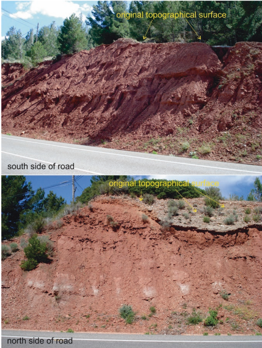
Fig. 11.2 Road cut slopes excavated in gypsum-cemented siltstone about 5 years after excavation. The slopes were excavated as a plane surface with a slope angle of about 60^\circ . The slopes are instable and eroded due to solution of gypsum after excavation. The north side is less affected than the south side, likely due to more direct sunlight on the north side and the pre-failing wind direction. The protrusive banks in the south side and greyish areas in the north side are layers mainly consisting of gypsum with little silt that are slightly more resistant to solution and erosion (Road C44 near Vandellòs, Catalunya, Spain)
