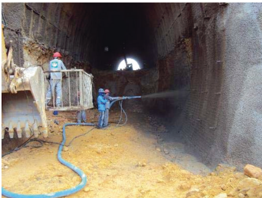
Fig. 5.18 Application of shotcrete and steel grid in bench walls (Photo E.L. Pastore)
