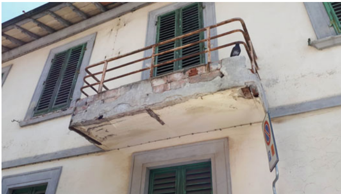
Fig. 3.1 A balcony photographed in 2019 near Florence, Italy. You can see the badly corroded iron beams appearing through the cracks of the concrete structure. This balcony is in a dangerous condition and it might collapse under stress but, apparently, the owners of the building cannot afford to have it repaired, a common condition for many reinforced concrete structures, all over the world. The pigeon, of course, does not care! (photo by the author, 2019)
