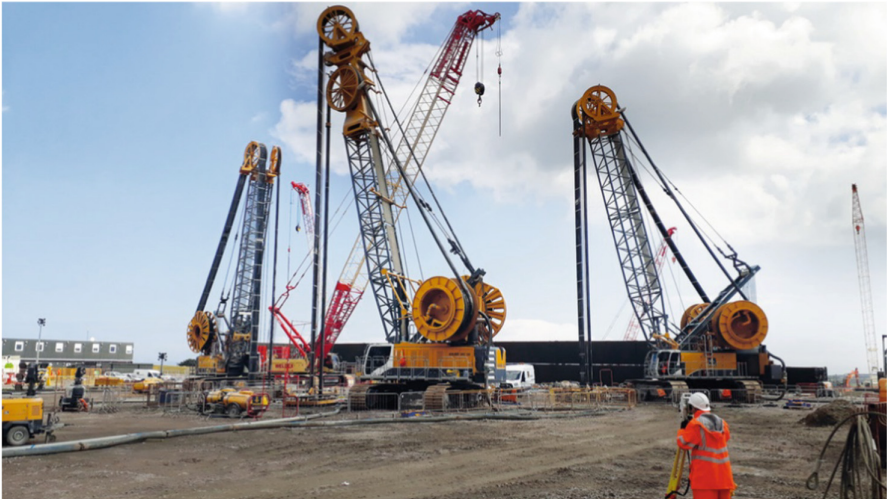
Fig. 2. Construction site with 3 cutters for the construction of a shaft in the UK (Quelle: BAUER)
