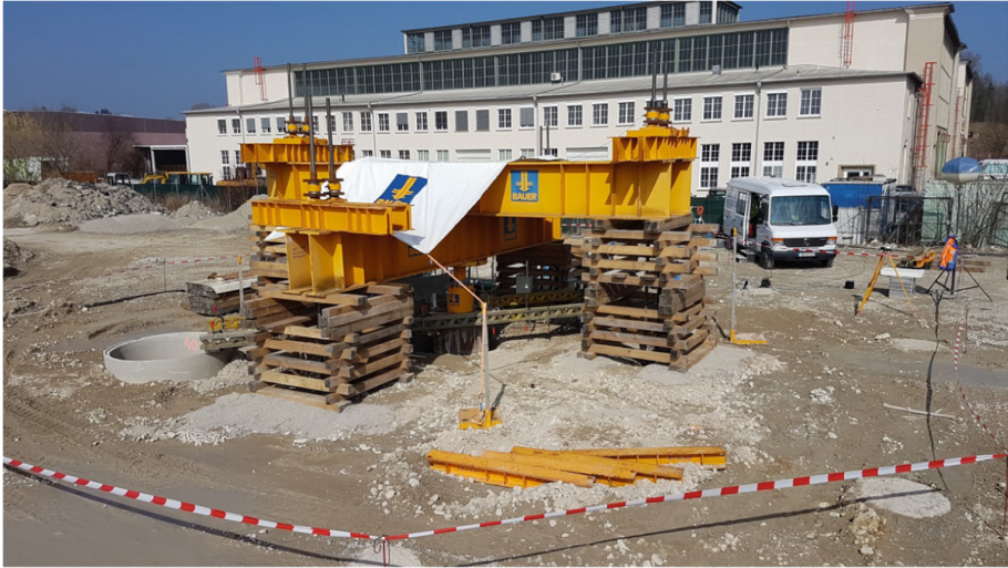
Fig. 8. Pile loading test (pile P10 is depicted) – load transfer beams and loading setup, vehicle containing the measurement equipment and a surveyor's dumpy level.
