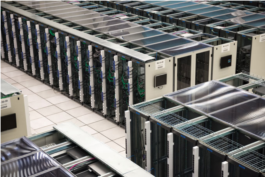
Fig. 16 CERN Data Centre
