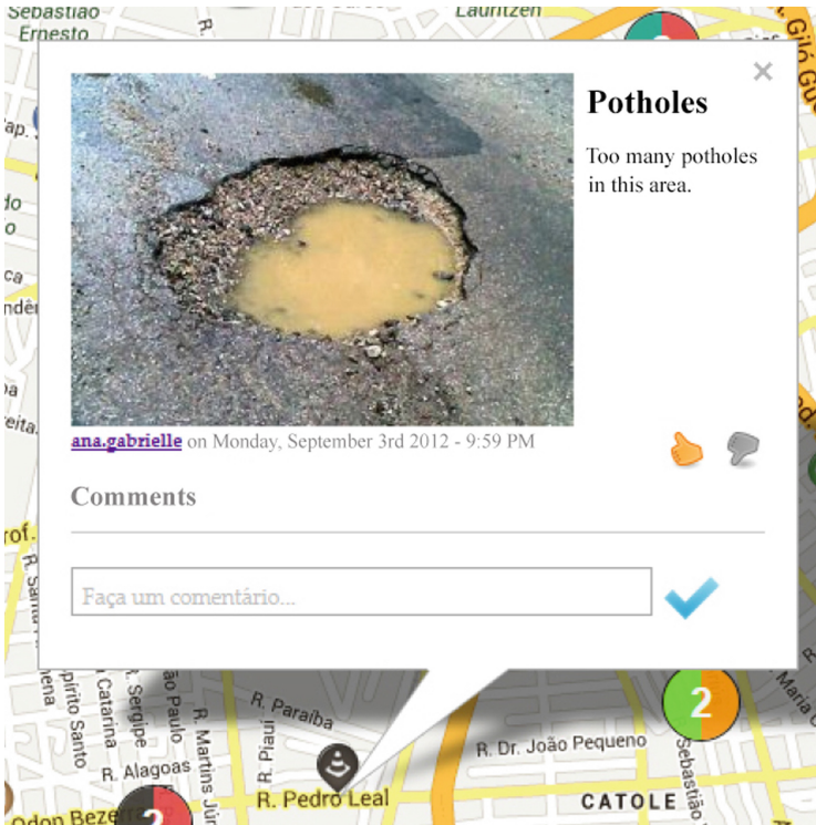
Fig. 3. A pothole complaint shared on the Crowd4City.
