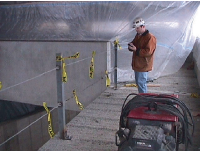
Fig. 14.2 A WVU Fall-Safe coordinator audits a guard rail at a Fall-Safe contractor's site. Reprinted from NIOSH Construction Compendium: Intervention , by the National Institute for Occupational Safety and Health, 2002
