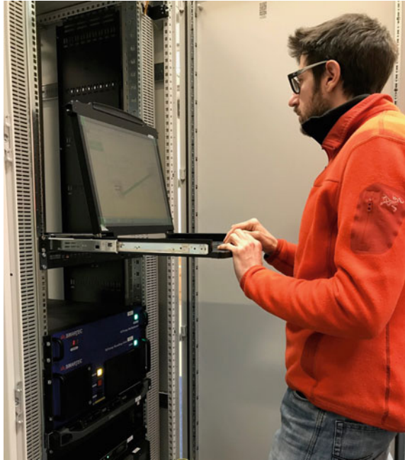
Fig. 12 Distributed temperature sensing system and ancillary equipment installed at pumping station
