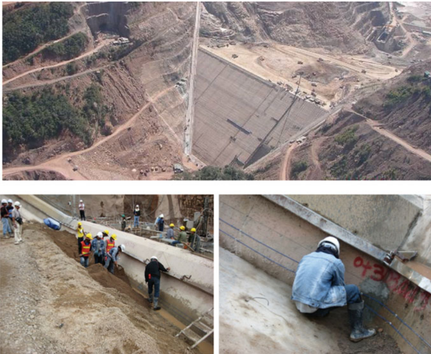
Fig. 13 Distributed temperature sensing cable installation along the plinth dam of the Nam Ngum Dam, Laos
