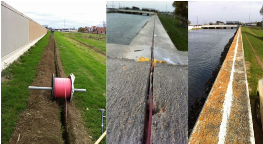
Fig. 17 Installation of distributed strain and temperature sensing cables in the levee foundations and on top of the I-wall and T-wall sections in New Orleans, Louisiana, USA
