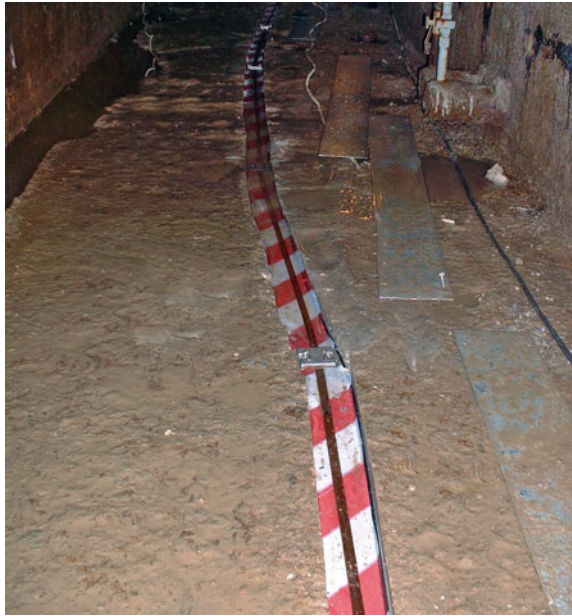
Fig. 22 Distributed strain sensing cable installed by clamping in the dam inspection gallery. The sensor runs along the length of the gallery and is therefore able to pick-up deformations generated by transverse cracks crossing its path. The blue temperature sensing cable installed along the strain cable is used for temperature compensation, but can also detect water ingress in the gallery by observing rapid temperature changes
