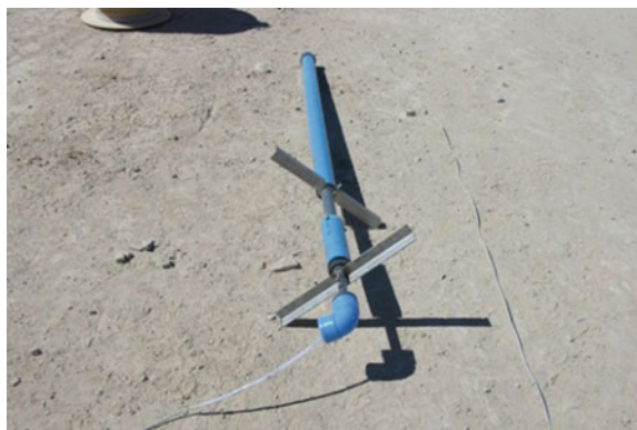
Fig. 31 Installation of long-gauge extensometers in the body of the tailing dam. Courtesy of Geomediciones
