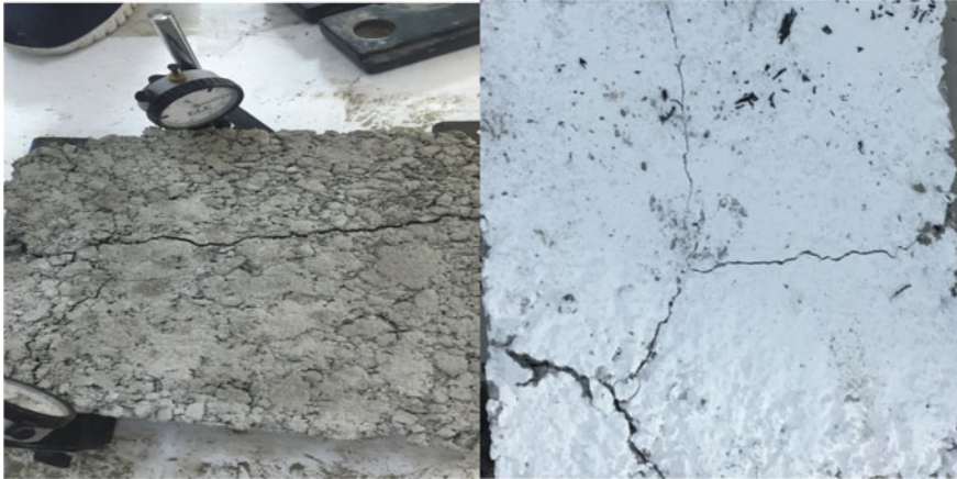
Fig. 1 Crack development on surface
