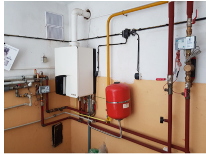
Fig. 2. Boiler room with heat consumption measurement for heating and hot water heating
