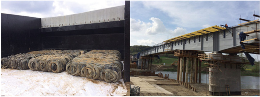
Fig. 8. Single layer of tyre bales before backfilling (left) and bridge construction (right).
