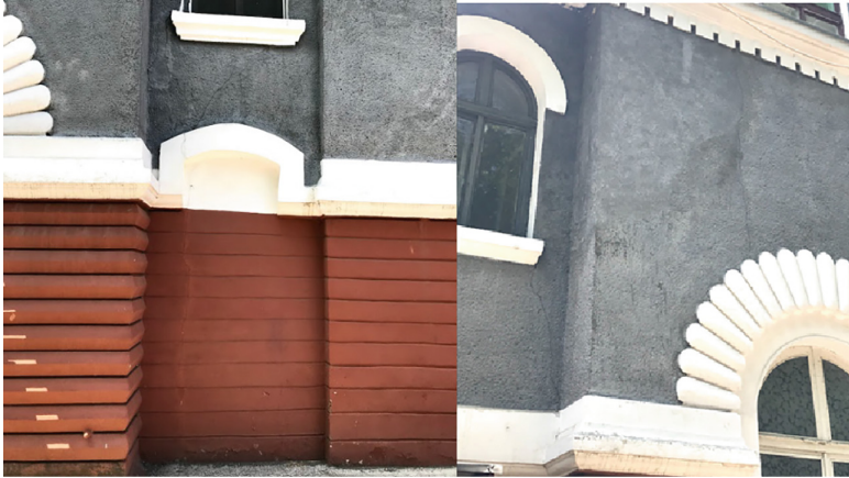
Fig. 3. Separate cracks above and below window areas
