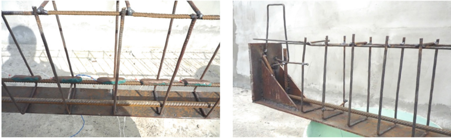
Fig. 1. Frames of steel plate reinforced concrete test beams with adhesion of steel plate reinforcement to concrete
