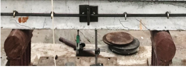
Fig. 3 Crack pattern on externally prestressed T beam using 12 mm diameter steel bars
