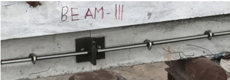
Fig. 4 Crack pattern on externally prestressed T beam using 12 mm steel strands
