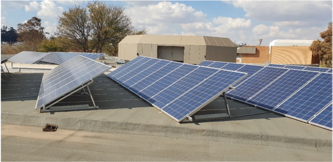
Fig. 3.9 Rooftop Solar at School of Business Leadership (Midrand) (Source: Author)
