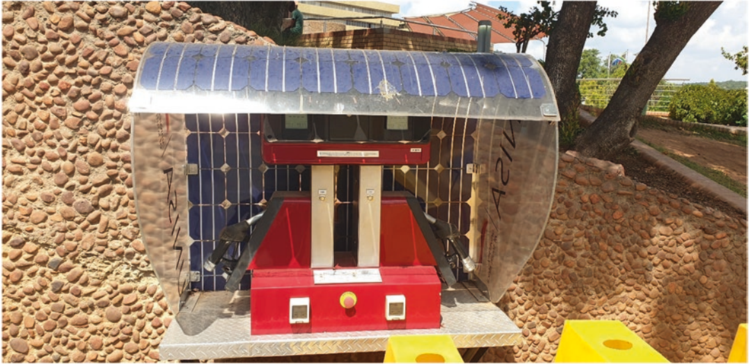
Fig. 3.15 Solar powered e-Vehicle charging station (Source: Author)
