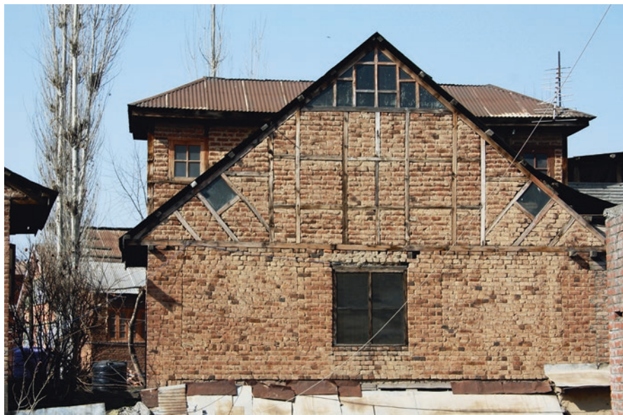
Fig. 9.6 Horizontal, vertical and diagonal bracing members in the upper section of the gable wall for improving out of plane performance
