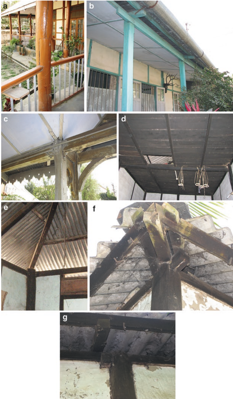
Fig. 9.14 (a) Splicing; (b) connection between vertical posts and horizontal rafters at verandah; (c) connection between vertical posts and horizontal rafters at eaves level; (d) connection between vertical post and wooden slab; (e) connection between vertical post, horizontal rafters and inclined roof member at eaves level from inside; (f) connection between vertical post, horizontal rafters and inclined roof member at eaves level from outside; and (g) connection between vertical post, horizontal rafters and asbestos sheet used for roofing
