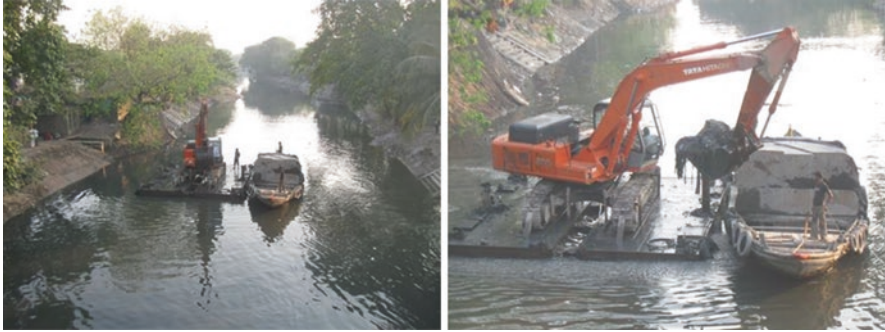
Fig. 11.5 Dredging in progress by the Irrigation Department, Government of West Bengal. (Source: Author 2012)
